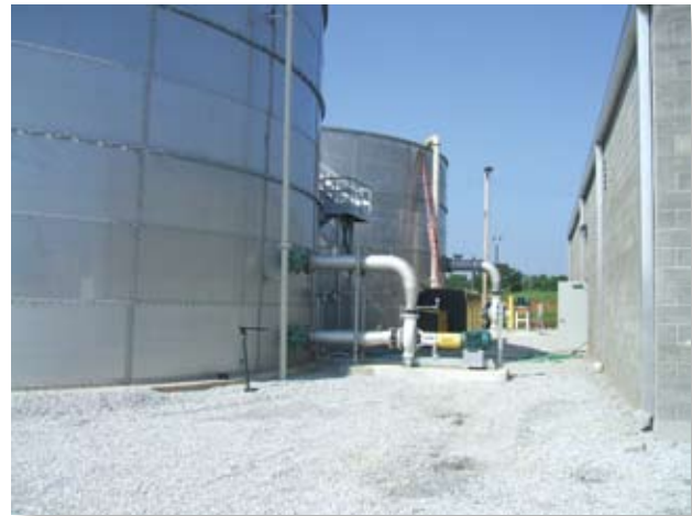
Design/build for General Mills by BCI to treat process water for non potable reuse.
