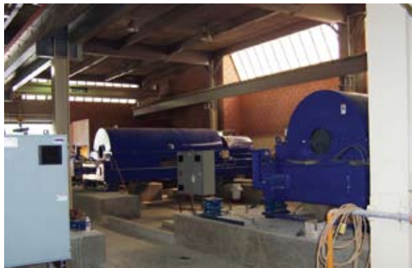
Metropolitan Sewer District of Greater Cincinnati Centrifuge
